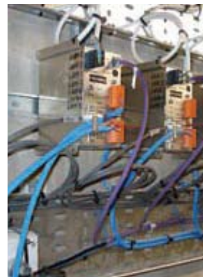
Central ECC control units for the AQUA3000 Open Water Management System
