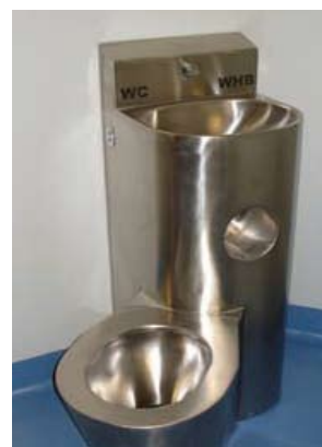
In cell sanitation unit with touch free water controls in Dublin Courts Building.
