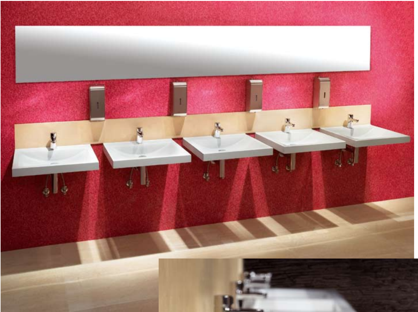
Multiple washing system with QUADRO single washbasins, AQUAMIX-C self-closing fittings and XINOX® Touch free soap dispensers
