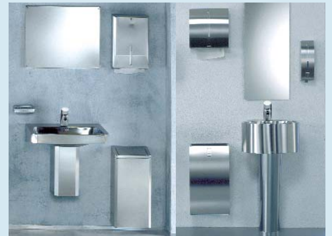
Various Franke product lines were installed in the washrooms of the O2 Arena in Prague: the VIP areas were fitted with the high-end Xinox range (picture above). The Chronos and Stratos ranges were used in the public facilities (photos below).
